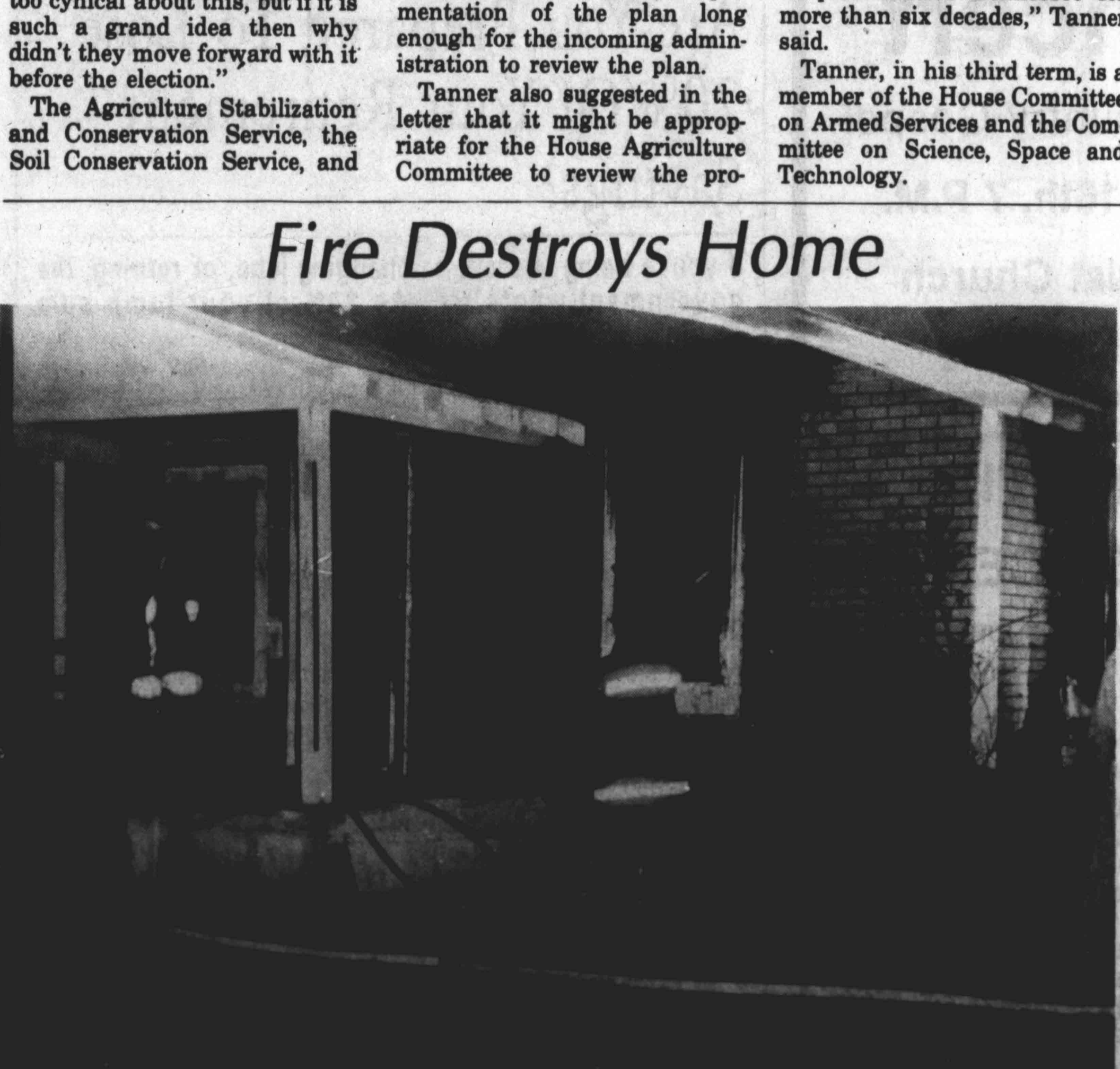
HALLS FIRE DEPARTMENT answered a call to a house owned by Mrs. Lucille Thurmond at the corner of Pearl and Sumrow Streets in Halls at 7 p.m. Monday. Occupied by Thomas Phipps, Mrs. Chantay Bostic and children, the house was gutted by fire. No one was at home at the time of the fire.
